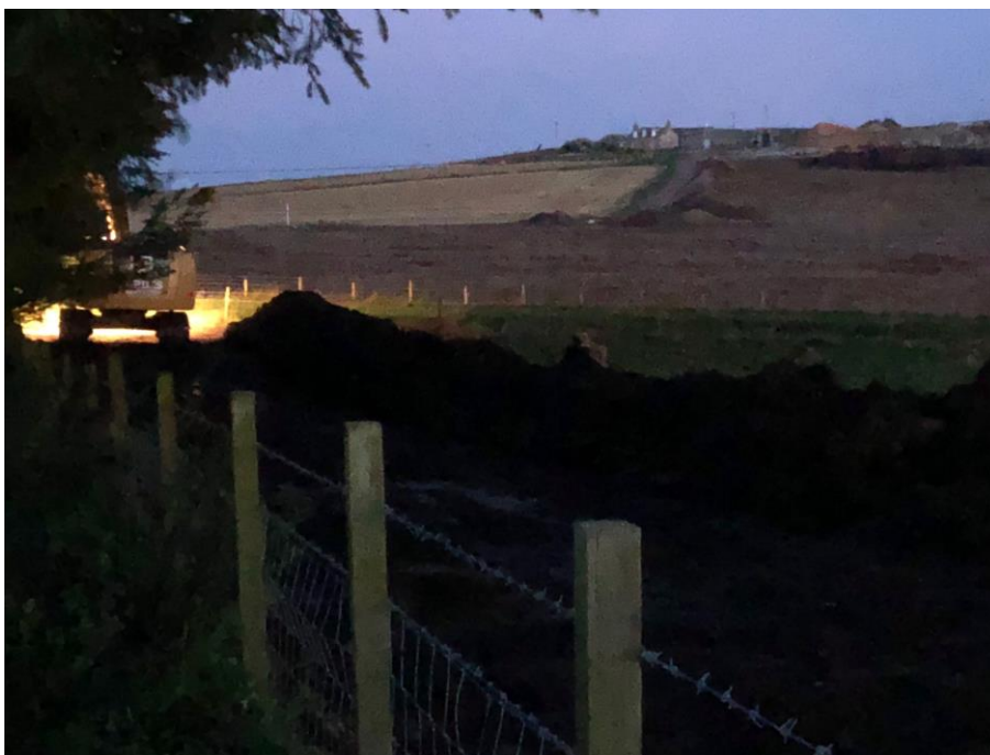
Figure 2 - Works being undertaken very early hours of the morning in September 2018. The applicant advises that these works were carried out by Forbes Homes Ltd, after the committee granted planning. Works included digging a deep trench severing and removing parts of all drains leaving Rothnick Croft.
